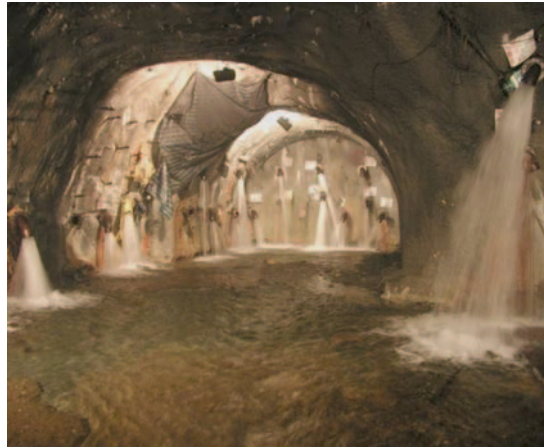
Fig. 10 New Yung Chuen Railway tunnel, continuous water inflow of approximately 500 l/s. The image was taken about four years after the catastrophic water ingress occurred in October 1998.
