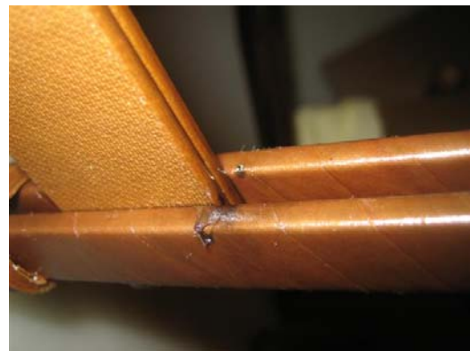
Figure 9: Creepage across the spacer edge and punctures on the two paper-wrapped conductors.
