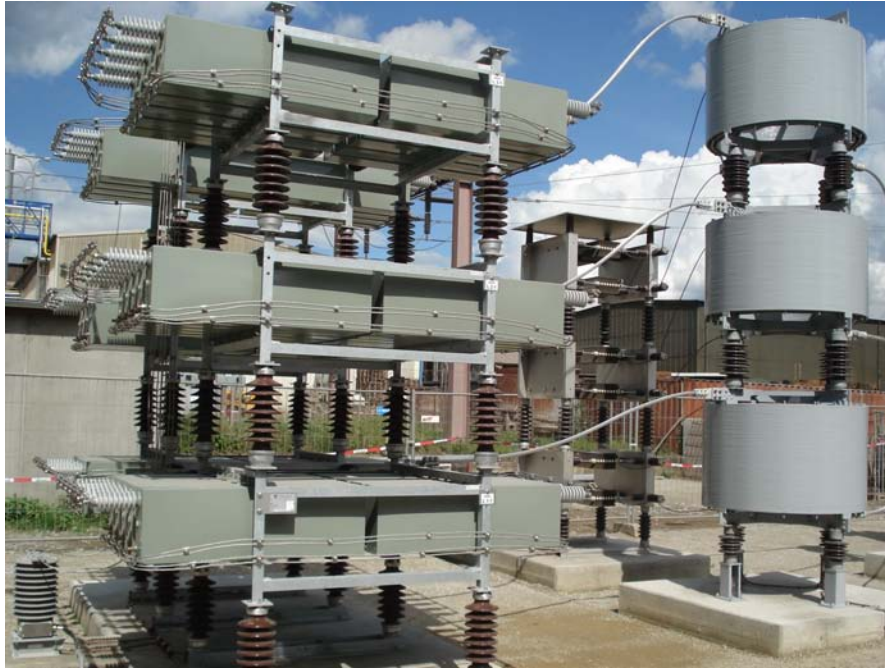
Fig. 5 Capacitor bank of SVC with series inductor
