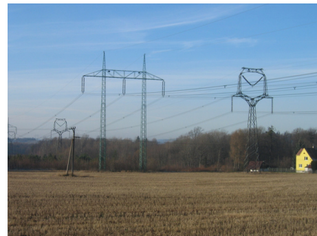
Fig 1. EHV overhead lines
