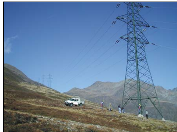
Figure 1: The studied, high alpine overhead line
