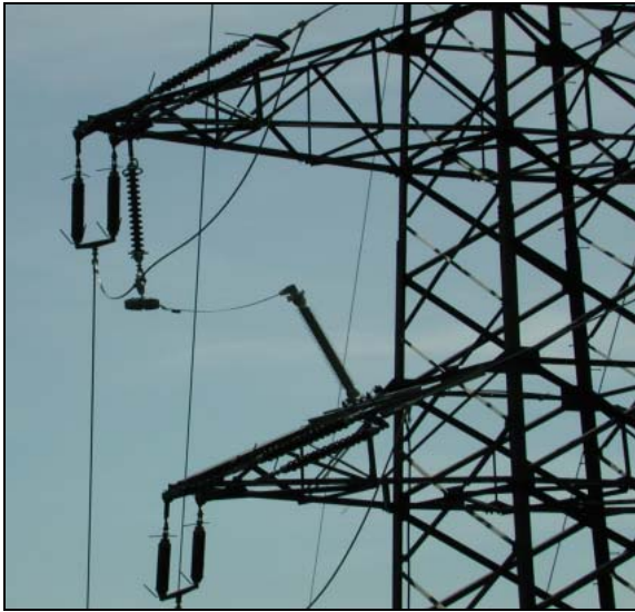
Figure 4: Application of a line surge arrester on a dead-end tower (arrester located at bottom cross-arm)
