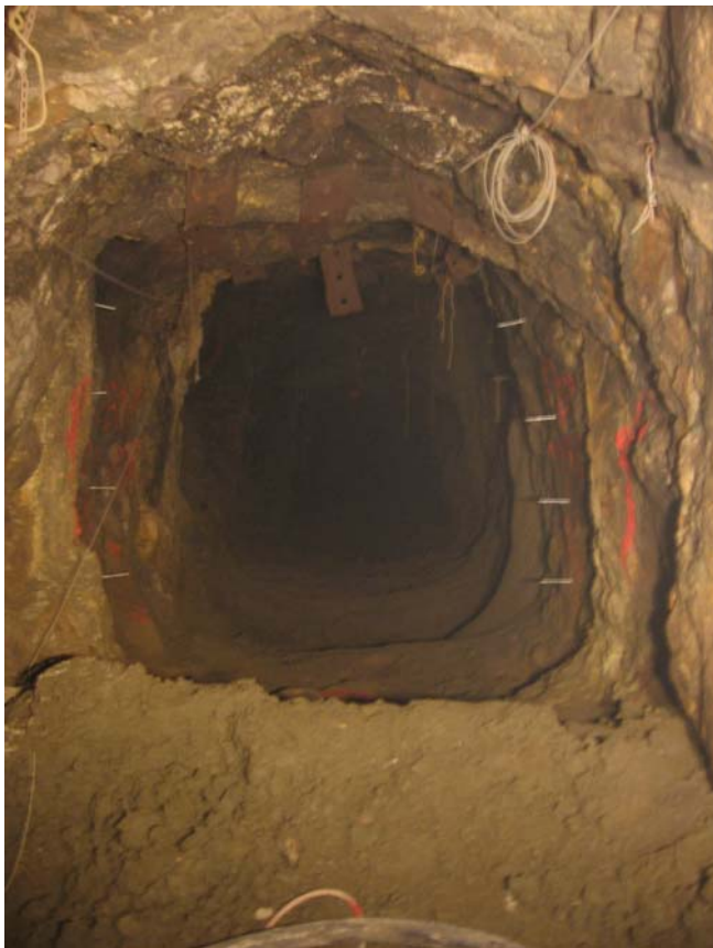
Fig. 4. Army Tunnel conditions prior to bulkhead construction (future bulkhead location indicated by sidewall anchor bolts).
