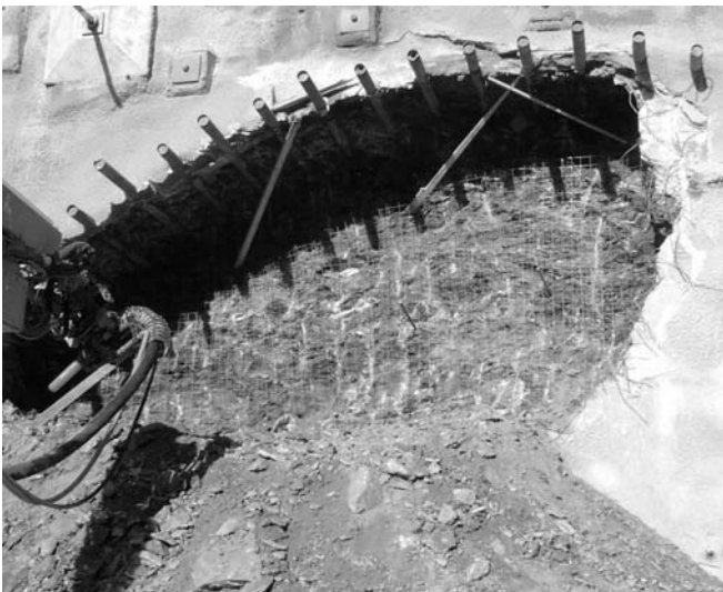
Figure 1. West portal of the Birgl tunnel (AUSTRIA) supported by a pipe roof
