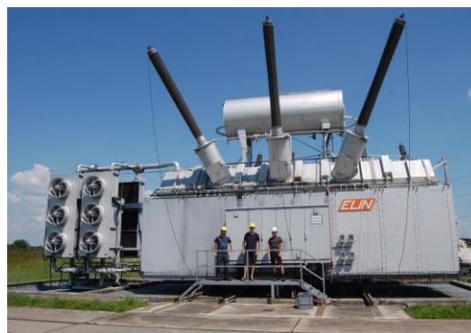
Figure 16: 5-limb 300 MVA power transformer
