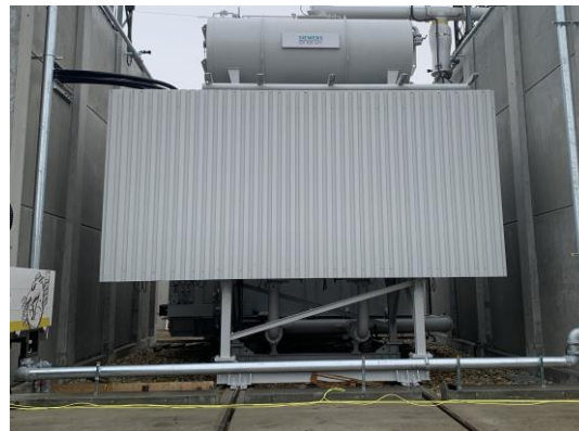
Figure 12: 2-limb 1-phase 183.3 MVA transformer
