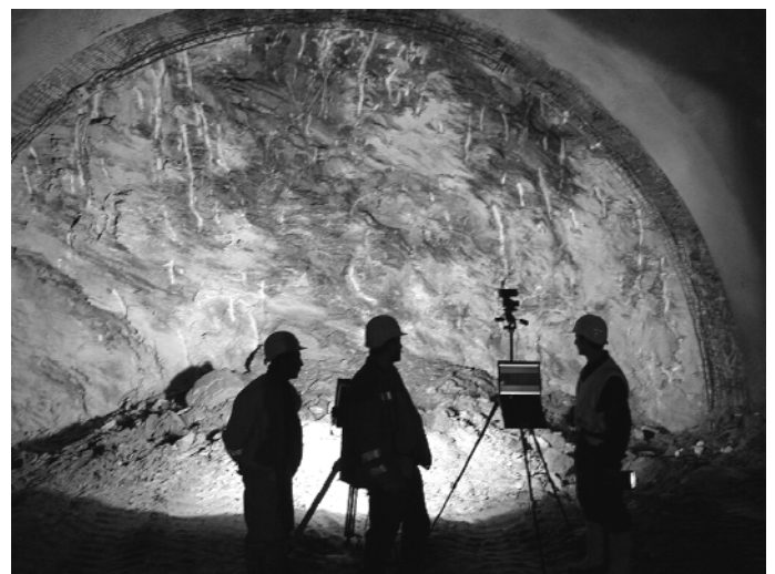
Figure 3: Imaging at the tunnel site. Note that only one person is required to operate the scanner.
