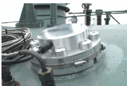
Fig. 5.2: Externally mounted UHF sensor on the tank of a 1000 MVA transformer [9]
