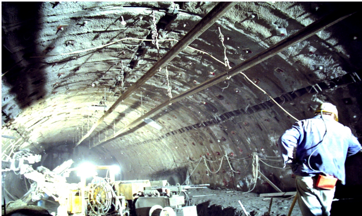
Figure 7. Three rows of yielding elements installed in the shotcrete lining at the Semmering base tunnel
